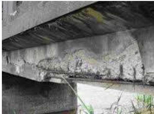
Figure 1. Damage to concrete structures due to corrosion.
